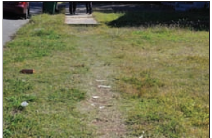
A path worn into the grass due to an incomplete or removed sidewalk segment in the 12th Street Core plan area.
