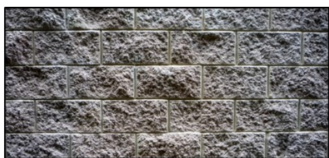
Figure 59. Split-face concrete block can be used as a foundation material to convey that even an replica in all other respects of a historic building is in fact contemporary.
