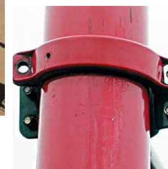
The clamp on this equipment is missing hardware which must be replaced.
