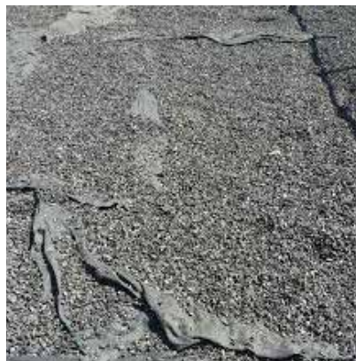
Geotextile fabric should never be exposed and is a sure sign that surfacing levels are inadequate.
