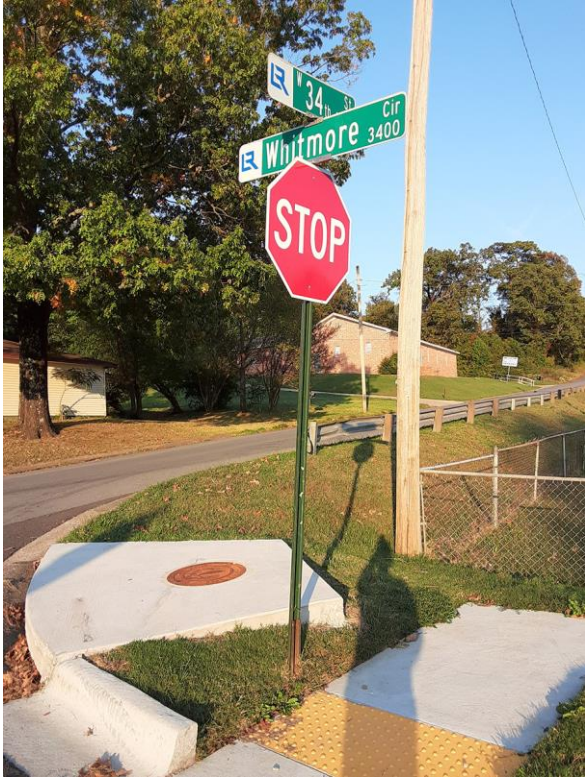
New storm drain facilities.
